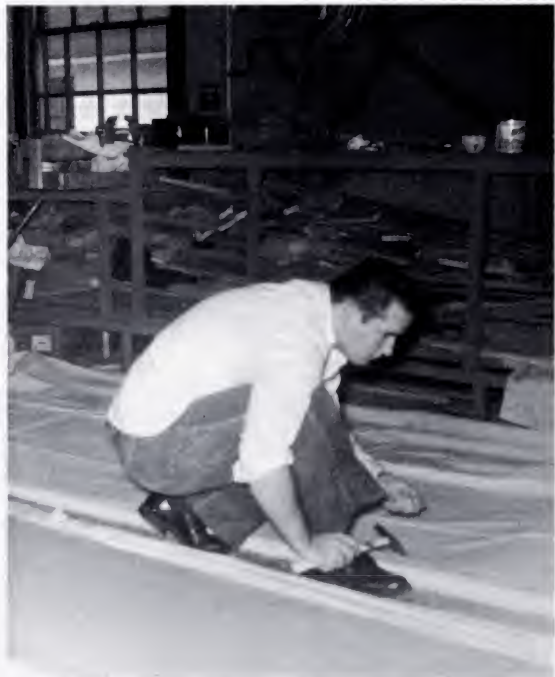
Below: Roni Eggleton is shown as he prepares to drive some nails in the building of the set.
